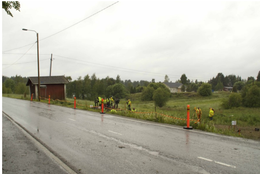
Image 12: Excavation work in Tursiannotko next to Anian rantatie. The group of people is located close to where they found evidence of a Viking Age house. Site visit on 29.07.2017.
