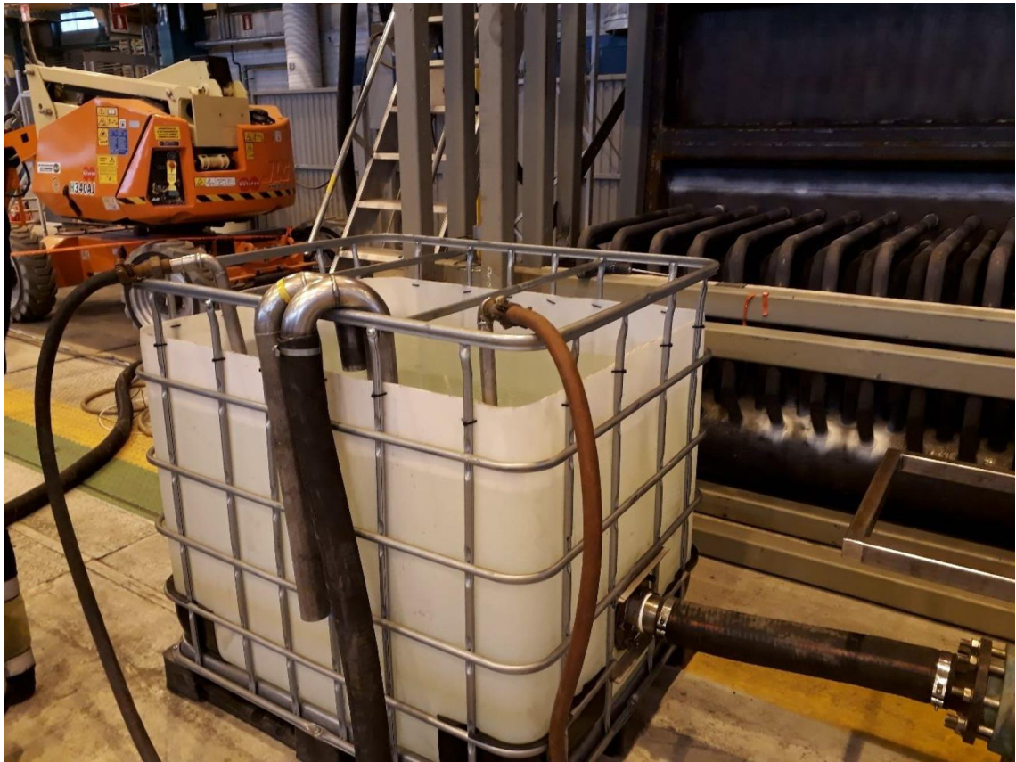
Figure 13. Chemical mixing pool.
