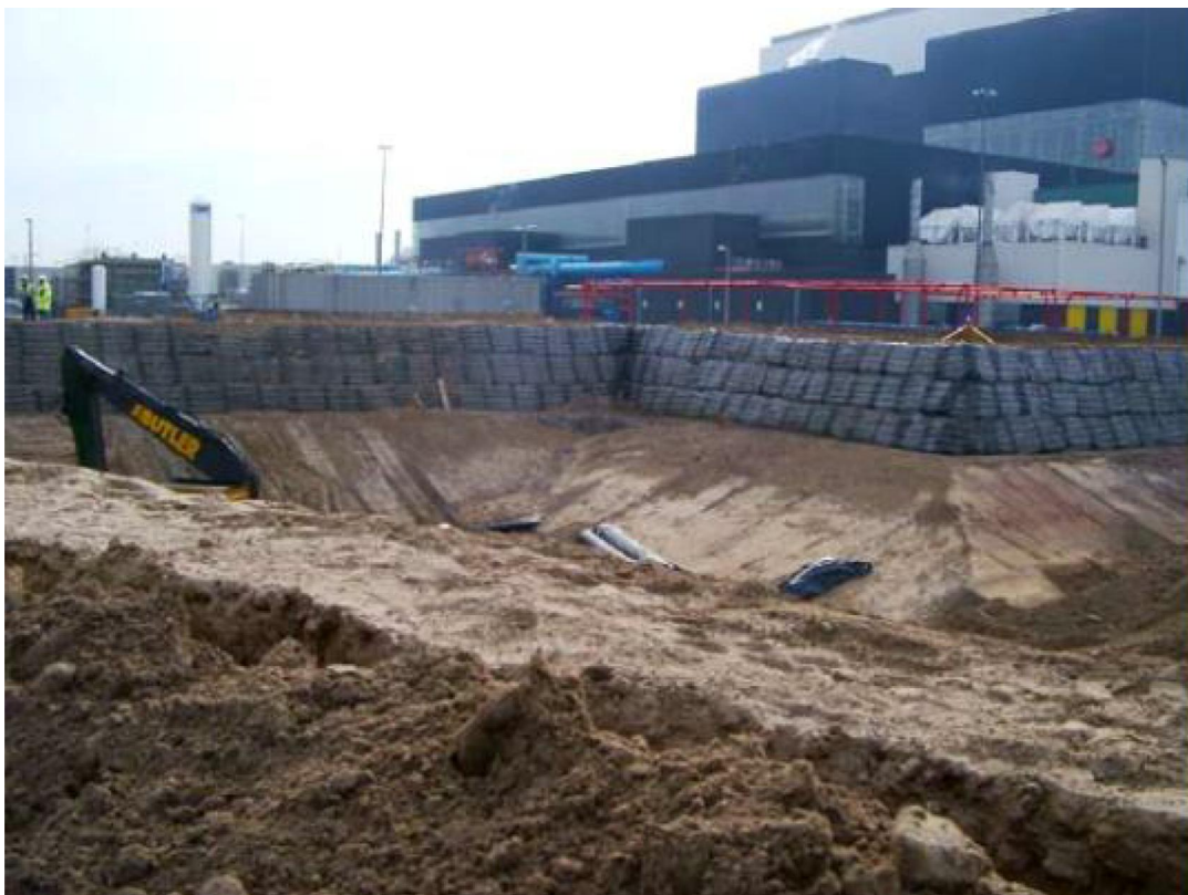
Figure 5. On-site pond for storage, neutralization and precipitation [37].
