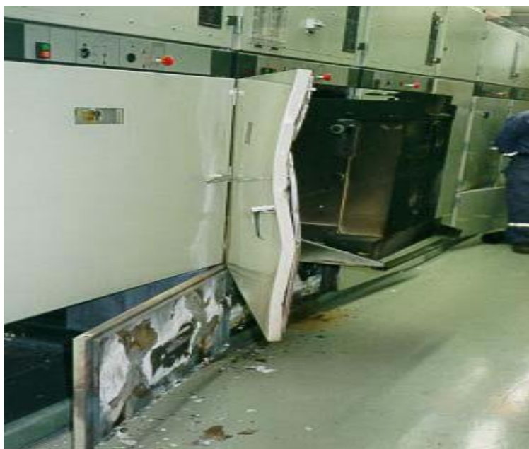
Figure 3.1 Arc short circuit effected Substation cabinet. Source: ([23])
