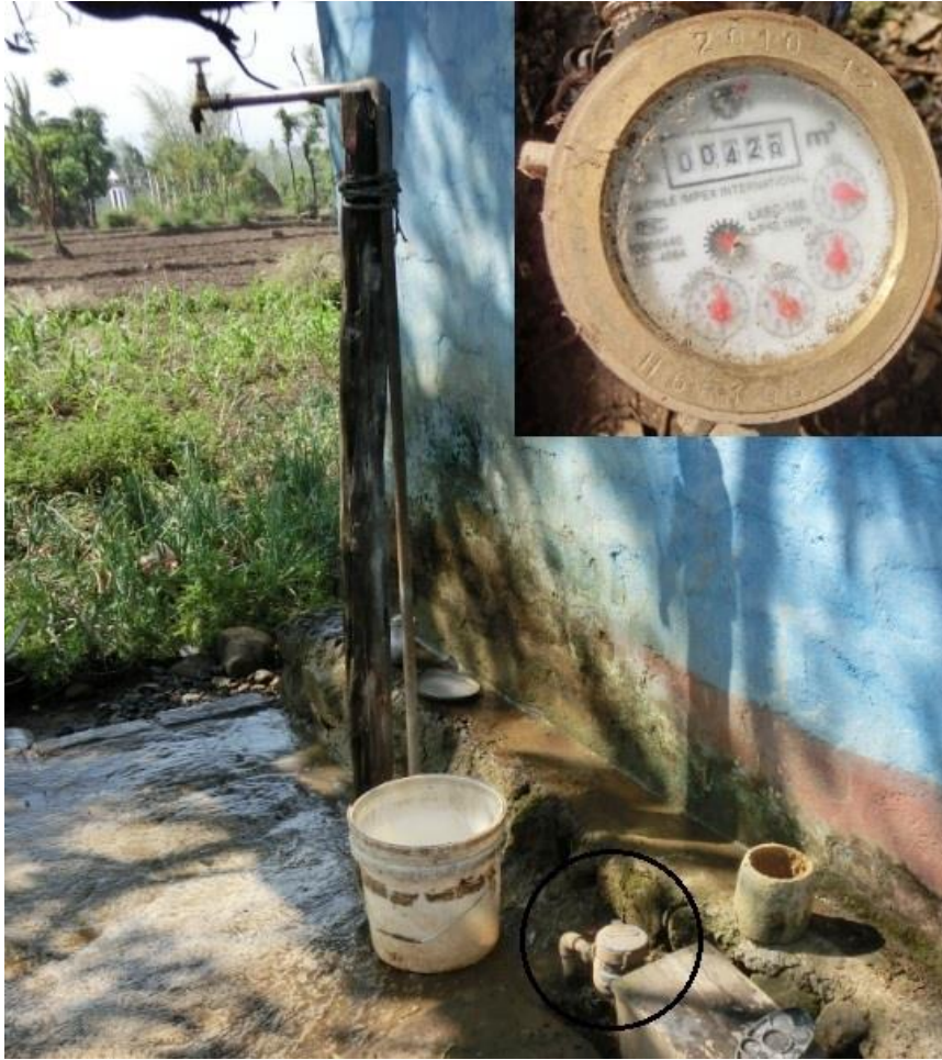
Figure 22. A private tap and a water meter (circled in the picture) in a yard in Aaptari.
