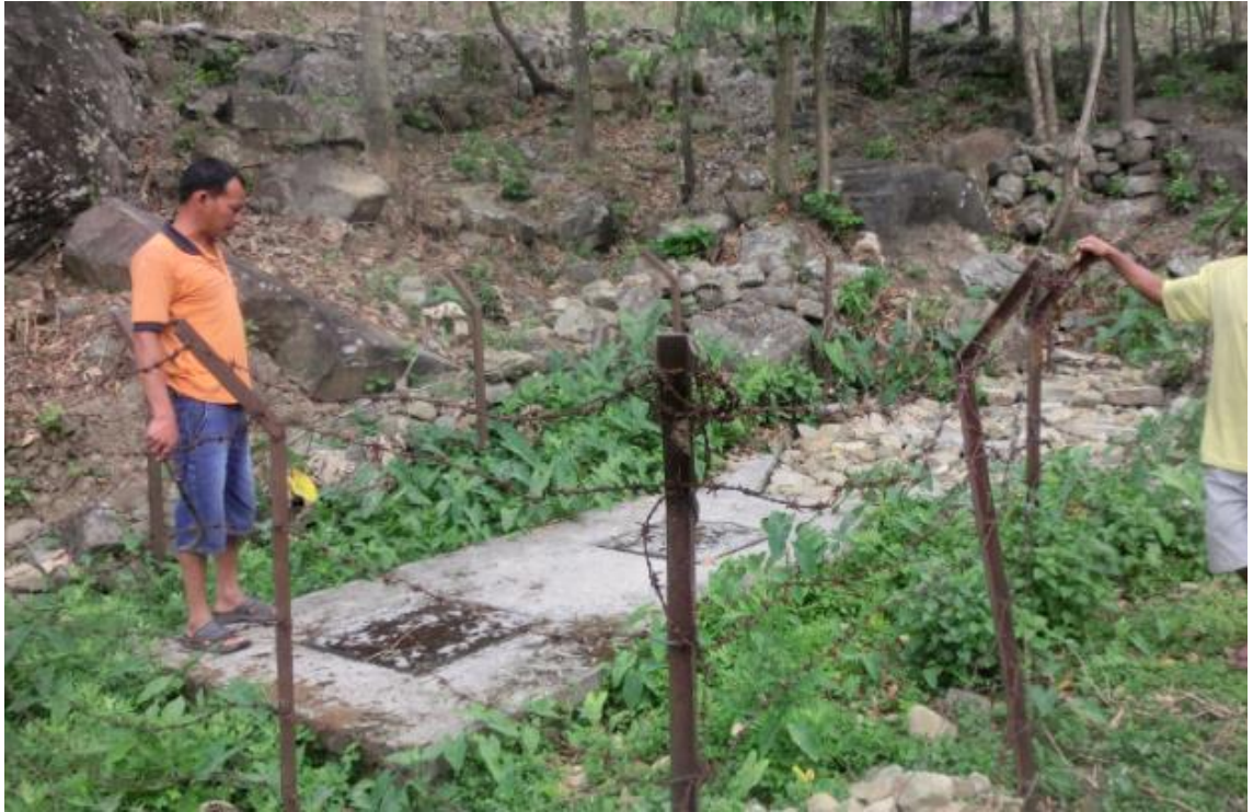
Figure 2. A spring intake in one of the visited villages, Kirtipur thulo gau. The spring (on the right) has been covered with stones to protect it. On the front, there are two valve chambers which are used to collect the water and pipe it forward to the reservoir tank.
