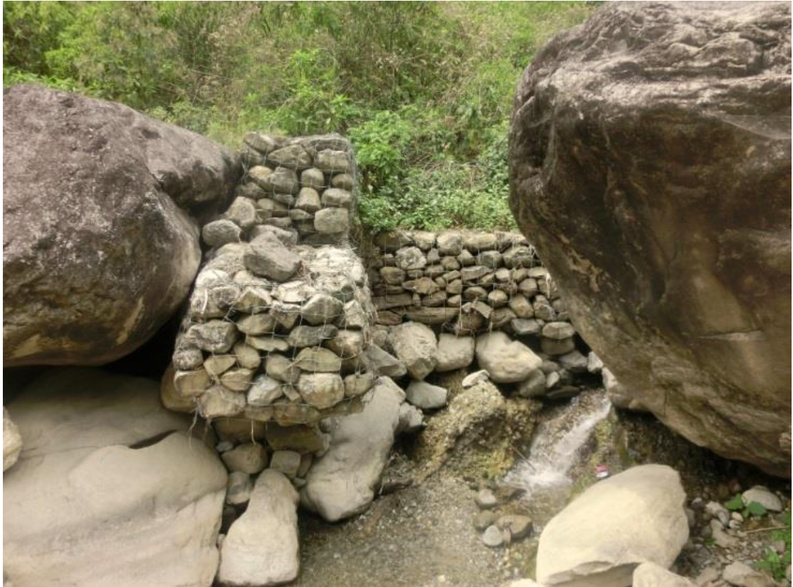
Figure 17. A typical gabion wall built at the source to cover it from flooding and landslides.
