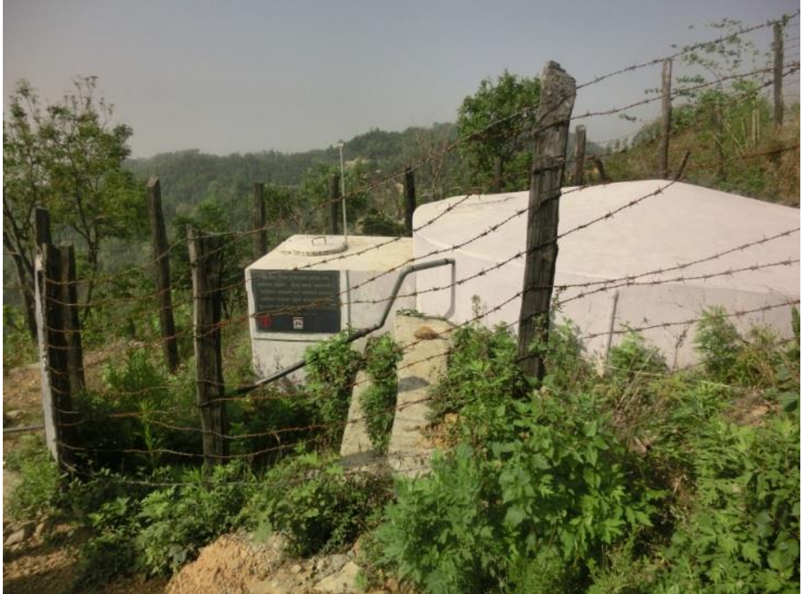
Figure 20. A new reservoir tank in Kumsot village, constructed in 2013.
