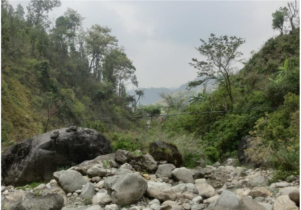
Figure 18. In the Chuhar scheme, the water source is located on the other side of the river, and the main pipeline has been installed in the air, crossing the river.
