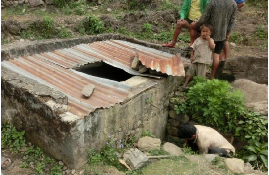
Figure 19. The reservoir tank of the Sangupari scheme.
