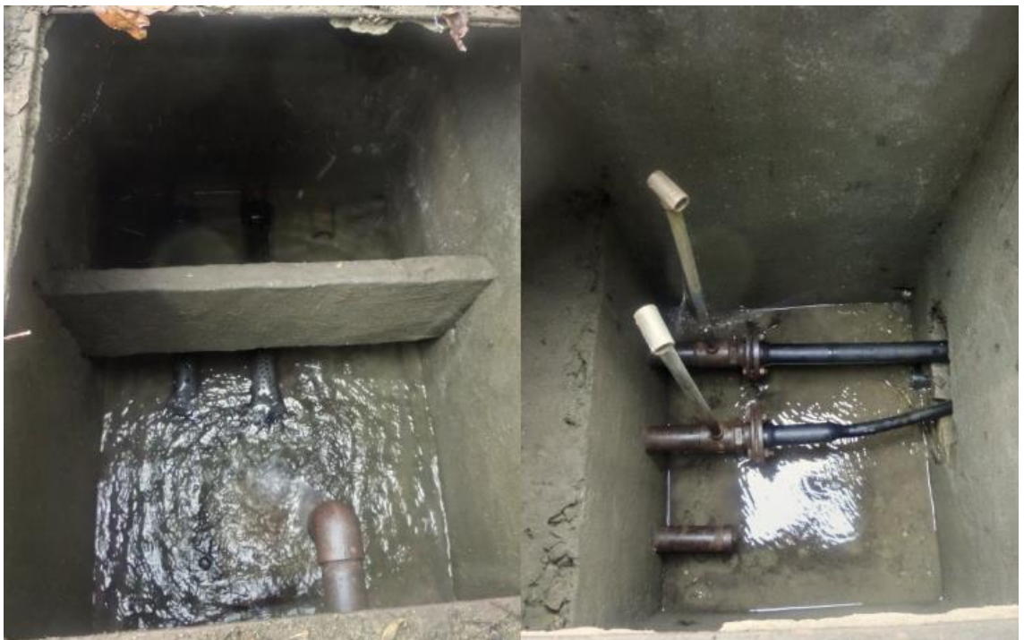
Figure 3. View from inside of the valve chambers at the Kirtipur thulo gau intake. On the left: the water comes from the spring to the first valve chamber from where the two main lines go to the reservoir tank. There is screening in the pipes of the first chamber.
