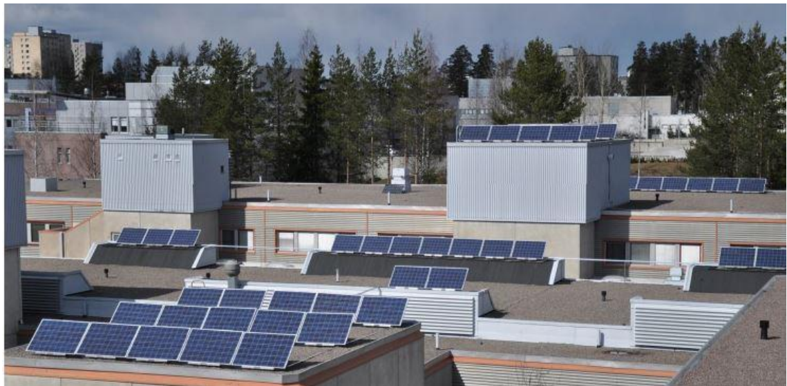
Figure 4.1 Solar PV power facility at TUT [24].
