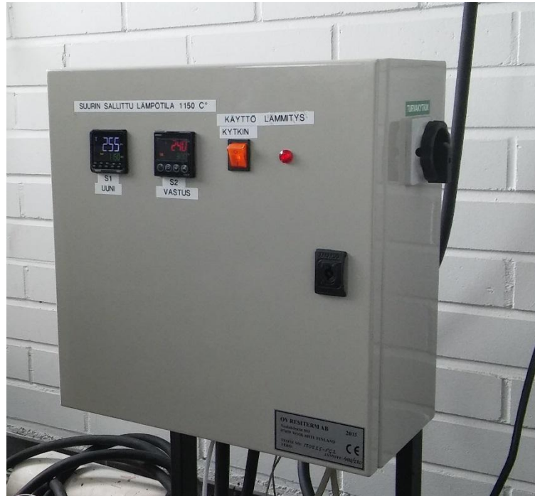
Figure 9. The oven controller unit.
