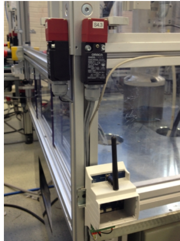
Figure 3.16: Door switch sensor connected to a wireless I/O sensor
