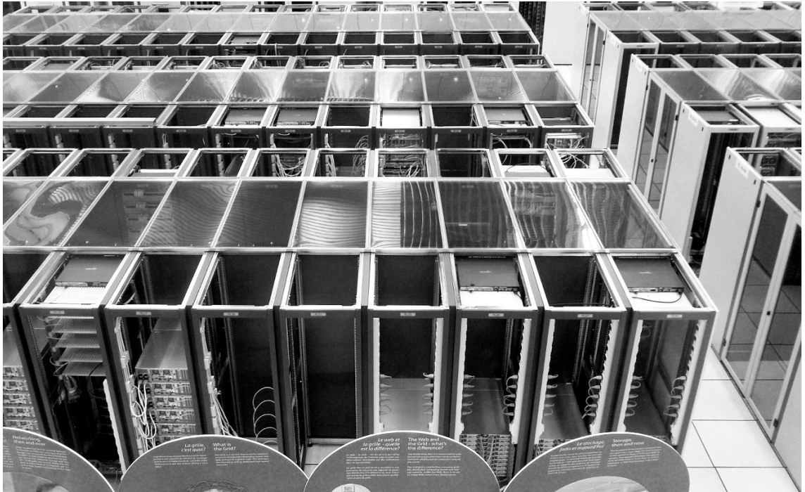
Figure 2.2: CERN computer centre. Some of the server racks are mostly empty because there is not enough cooling power to accommodate more computers.
