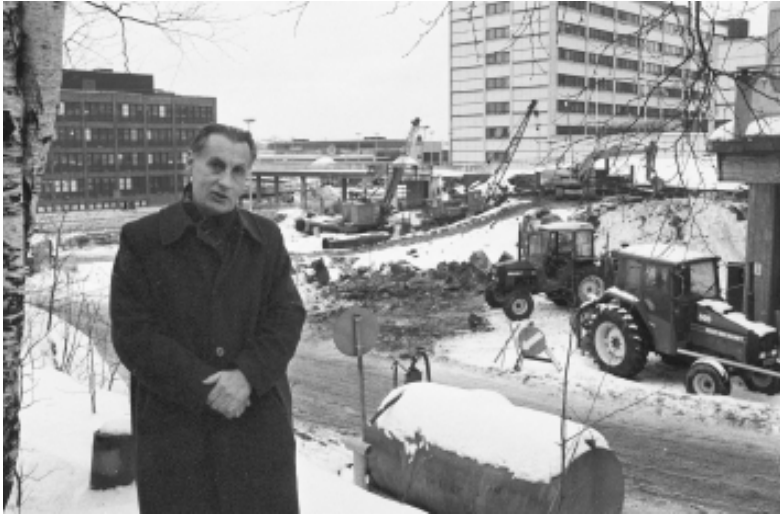
Professor Sven Hirn, at that time head of the library, in front of the construction site of the new Helsinki Main Library in 1984. The building was completed in 1986.
