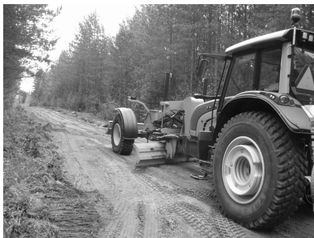
Fig. 3 A road grader was used to shape the road surface and mix the ash and aggregate
