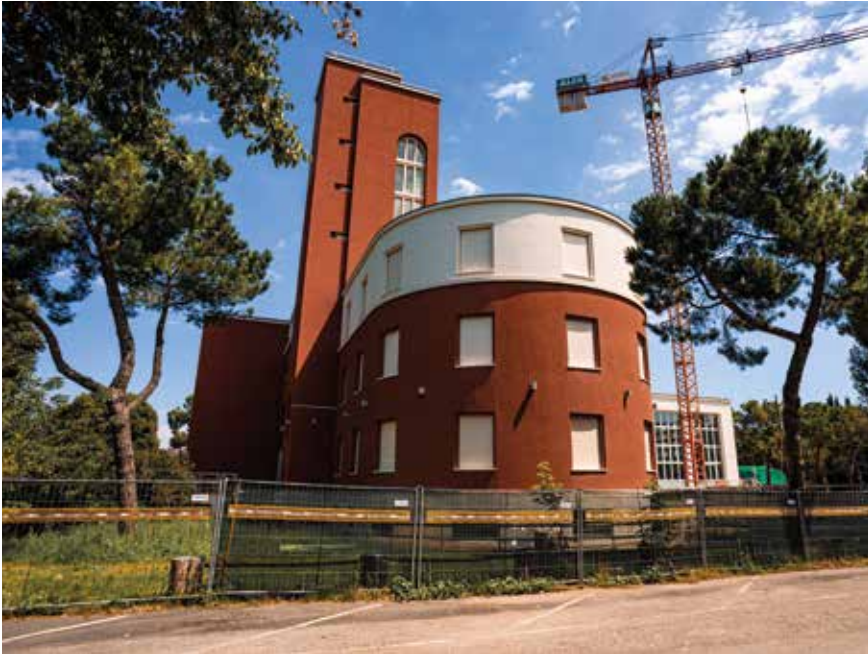
Figure 3. The headquarters of Opera Nazionale Balilla (ONB) under restoration in August 2014. Picture by G. Casa.
