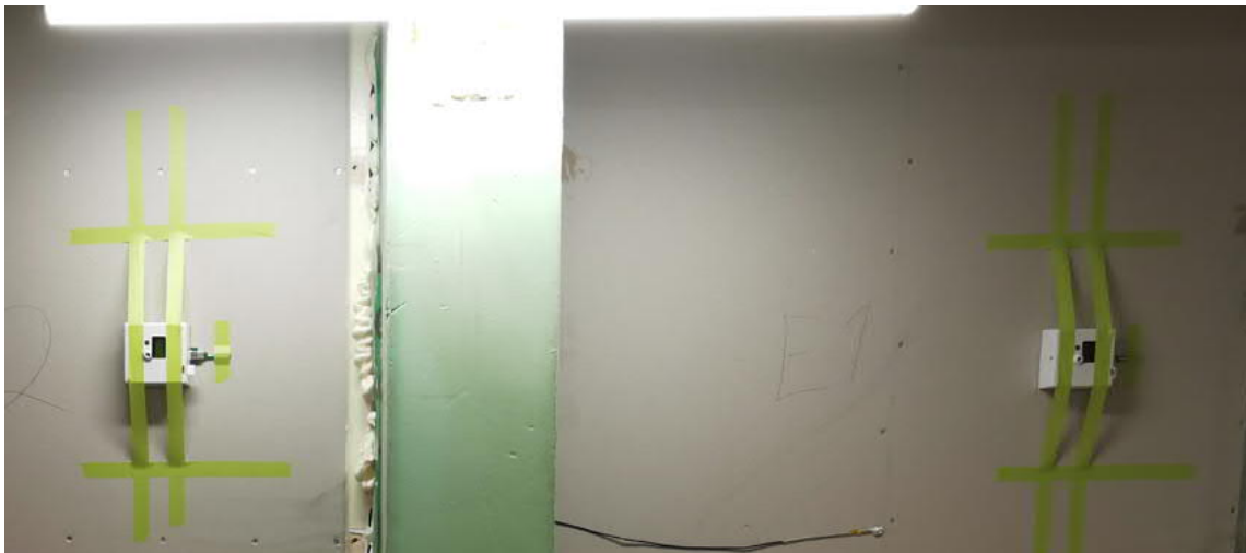
Figure 3. Two devices for rapid in-situ U-value measurement attached to test walls with adhesive tape.
