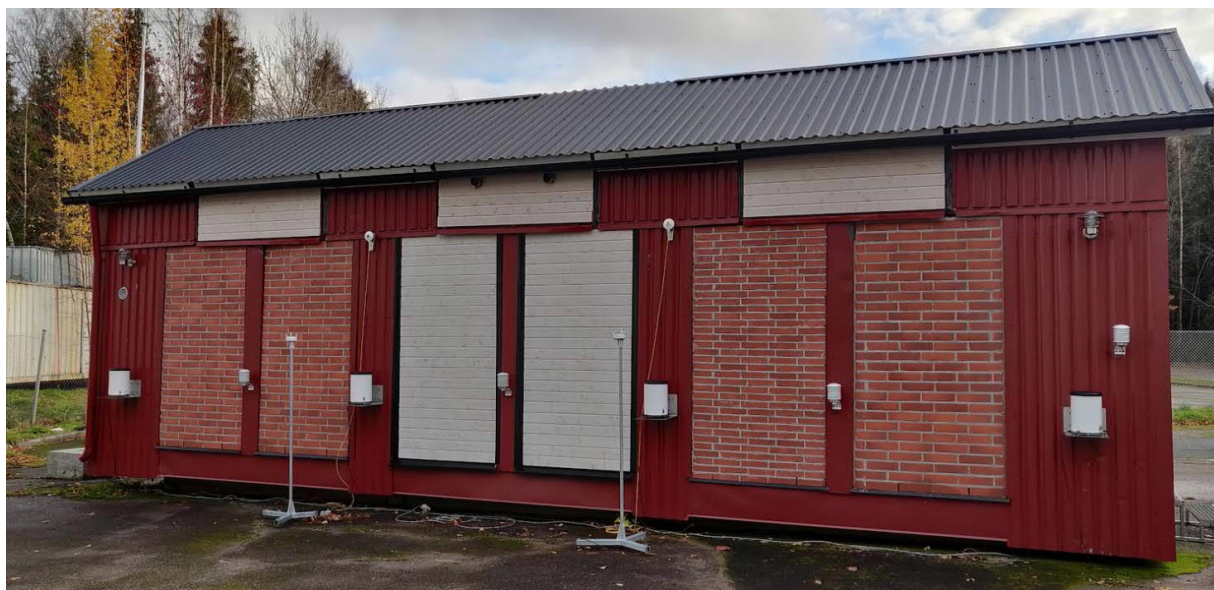
Figure 2. North side of the building physical test building in Tampere, Finland, with six test wall structures installed in the test openings.
