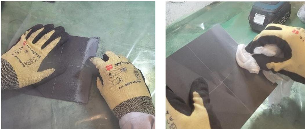
a) Sanding of laminate to Baseline level b) Removal of sanding dust
