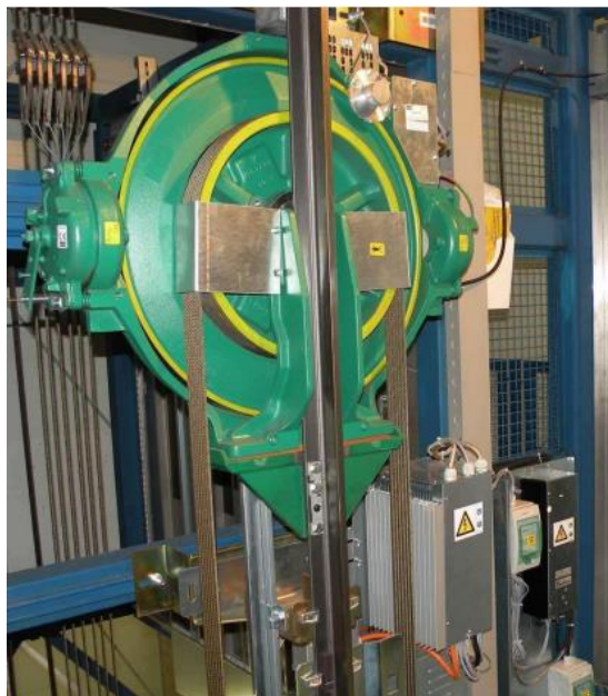
Figure 12. PMSM hoisting machine mounted on the elevator shaft wall [15]
