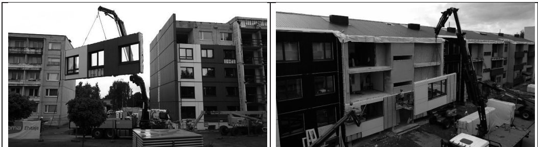
Figure 3. Renovation of 5-storey apartment building by using prefabricated insulation elements: MoreConnect pilot (left, [15]) and DRIVE0 pilot (right, [16]).
