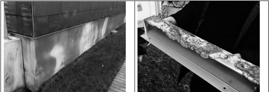
Figure 2.3. (a) Water drops containing chloride ions run down the vertical MgO-boards and drain out of the wall from behind the wall's siding boards; (b) Zink covering of the steel profile is corroded as a result of direct contact with salty leaked water from the adjacent MgO-board.
