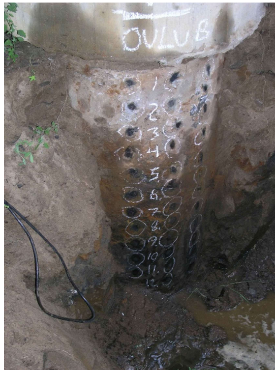
Figure 1. Bridge O-1684. Pile is cleaned and measurement points are marked. Steel pile is visible for 1.2 m below concrete column.
