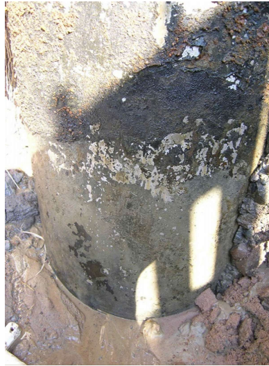
Figure 3. Excavation T-2436 and pile surface: on the upper part of the image can be seen corrosion on the pile surface in the man-made soil region, the surface inside the subsoil is remained in uncorroded state.
