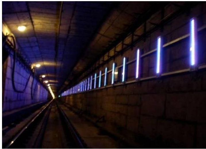
Figure 3. LED pillars on the wall of Shanghai's metro tunnel [26].
