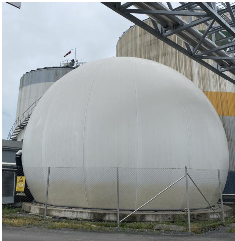
Figure 7. Gas holder at co-digestion plant. (Photo: Jancarlo Rodriguez)
