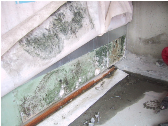
Figure 9. An example of a building structure with a double wind barrier attacked by mould growth on the board-based wind barrier.
