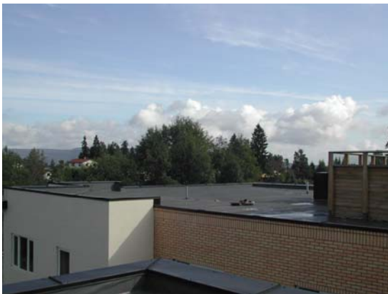
Figure 6. The roof of a public health building, one of the 12 roofs investigated.
