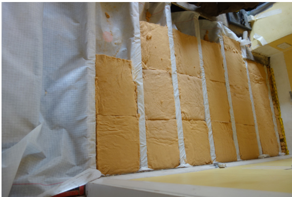
Fig. 4. Installation of woodfibre insulation in between the joists, held in a breather membrane over and under joists.
