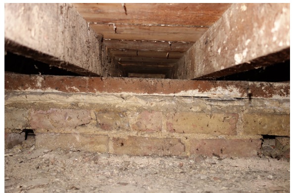
Fig. 6. A typical sleeper wall, showing also the openings between the joists, which were filled with insulation and hence leading to significantly reduced airflow between different floor sections.
