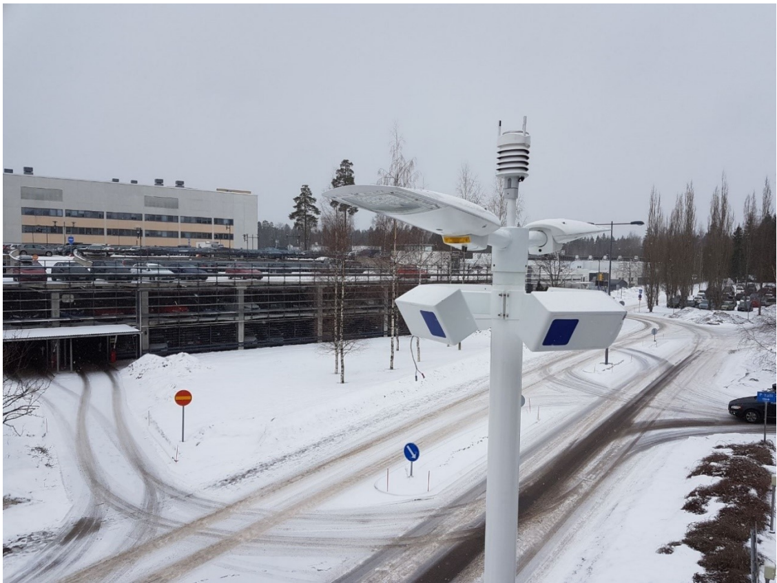
Figure 3.26: The position of the camouflage radome unit (CRU) in the light pole.
