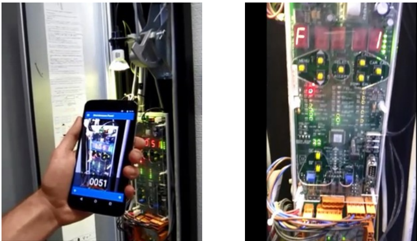
Fig. 4. The demonstrator: On the left, mobile application, (Fault 51 detected). On the right, image of detected maintenance panel with LEDs recognized.
