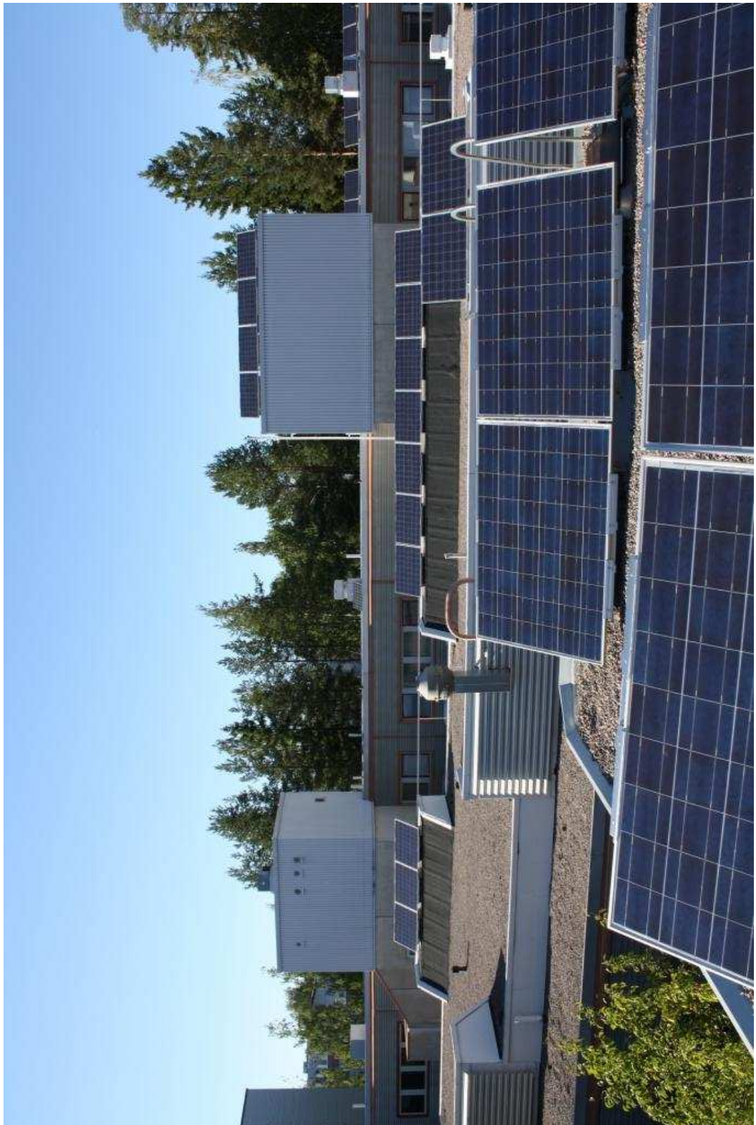
Figure B.6. TUT solar PV power station test plant I.
