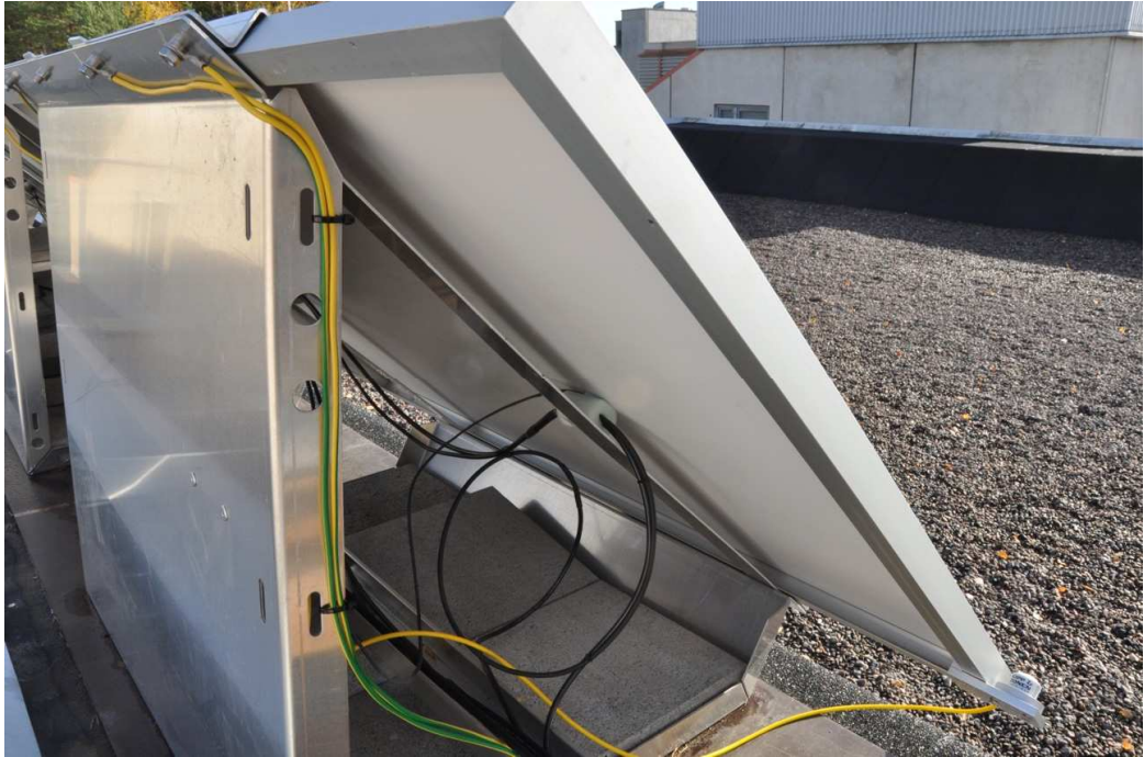
Figure 6.2. Platinum RTD attached to the back-side of a PV module.
