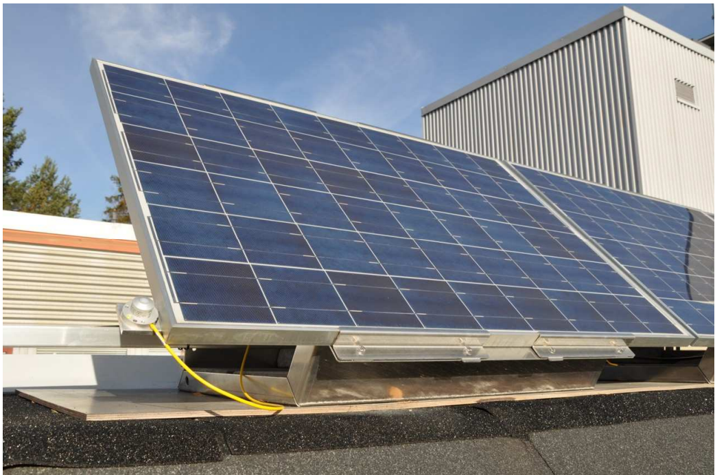
Figure 6.1. SP Lite 2 pyranometer mounted next to a photovoltaic string.
