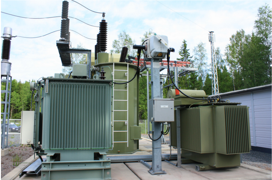
Figure 4.3 An earthing transformer (left) and the Petersen coil (right). Between the neutral point devices a disconnector.
