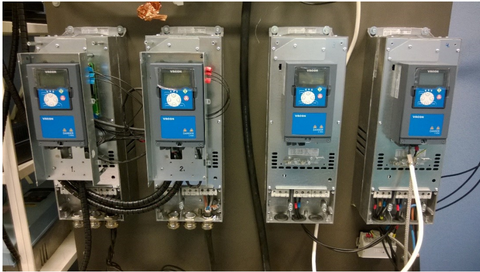
Figure 3.3. Vacon NXP converters. The first two from left side are generator side converters, the two in the right side are motor side converters.
