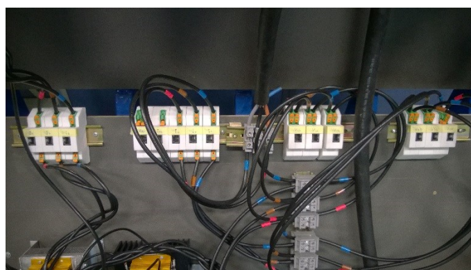
Figure 3.10. Installed current and voltage sensors.
