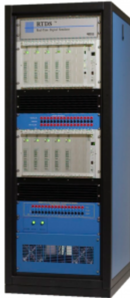
Figure 4.3 A mid size RTDS cubicle with two racks of cards. [20]
