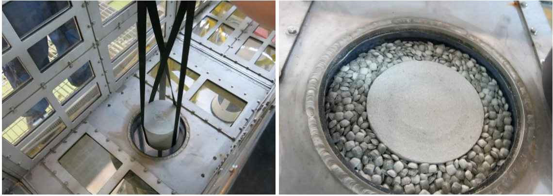
Figure 35. The buffer blocks were installed into the tube by straps and they were centered with the help of custom-made wooden sticks. The blocks and the pellets were installed in turns so the pellets stabilized the blocks that were already in the tube. The level of the top of the uppermost block was 30 mm below the tunnel floor level.
