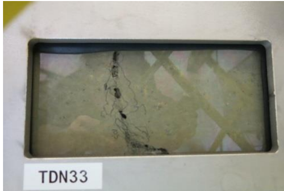
Figure 52. A water path in the window TDN33.
