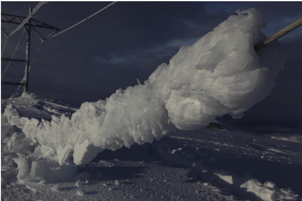
Figure 9. Rime ice accretion on the collapsed overhead line, Ålvikfjellet, Norway. [32]
