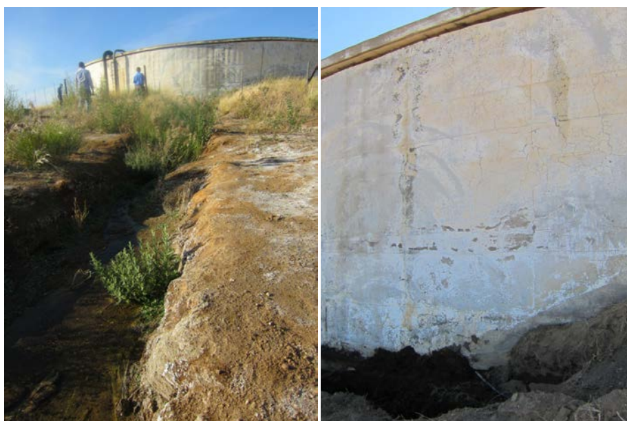
Figure 6.4. Leaking water reservoir at Donkie Draai (Tuovinen)
