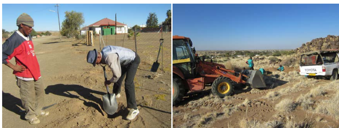
Figure 6.7. Finding leaking pipes is very time consuming (Tuovinen)
