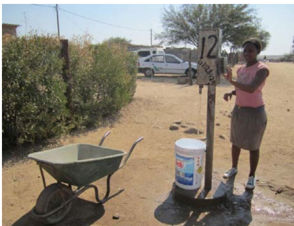
Figure 5.3. A woman using standpipe prepaid water meter (Saes, 2012)
