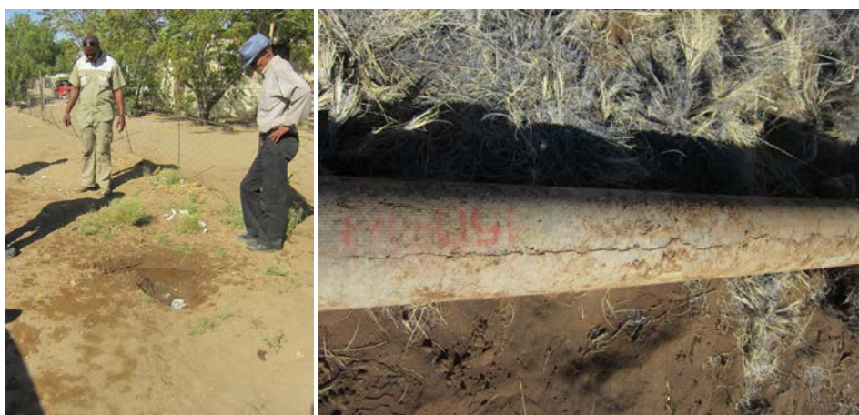
Figure 6.2. A visible leak on the ground (left) and an old leaking asbestos cement pipe with a typical fracture (right) (Tuovinen)
