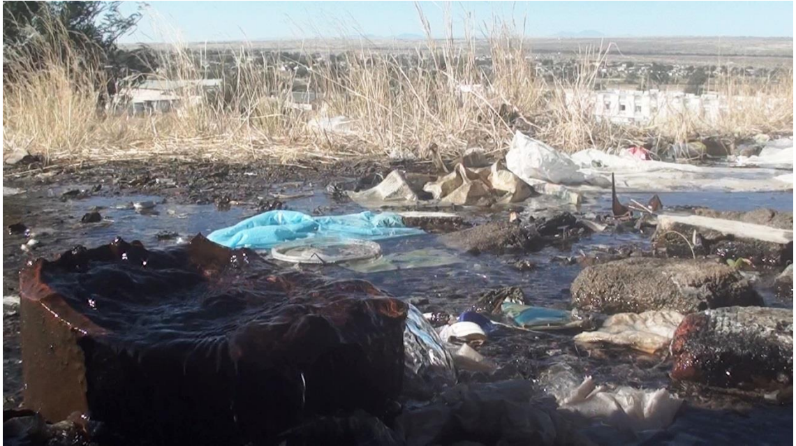
Photo 5. A leaking valve on Canon Cop hill. It was possible to measure the water loss caused by this leak by a cup and a stopwatch.
