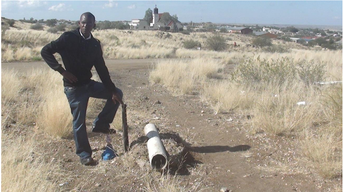
Photo 2. A new valve clearly marked with a metal post. Pipes are not deep and the valve is almost on ground.
