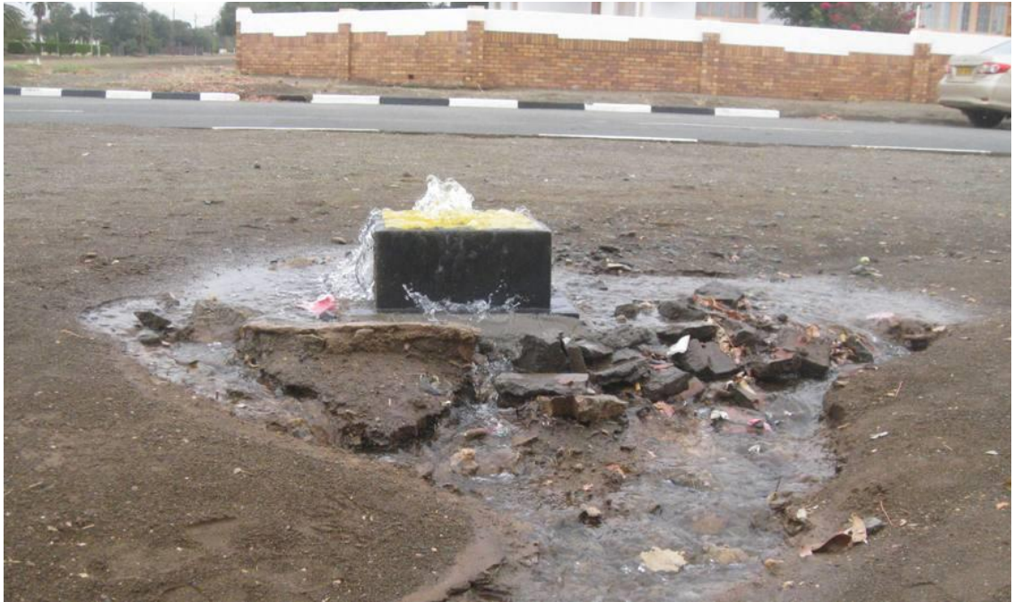
Photo 1. A Fire hydrant opened for reducing pressure to help fixing a leak nearby. The leaking pipe was not possible to close by valves. (Photo: Pekka Pietilä)
