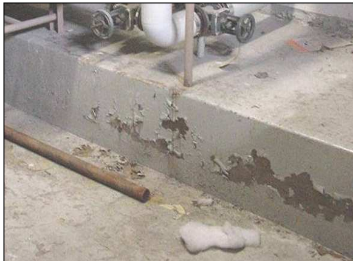
Figure 2: Flaking PCB-containing paint from a school building (Kuusisto et al. 2006-a)
