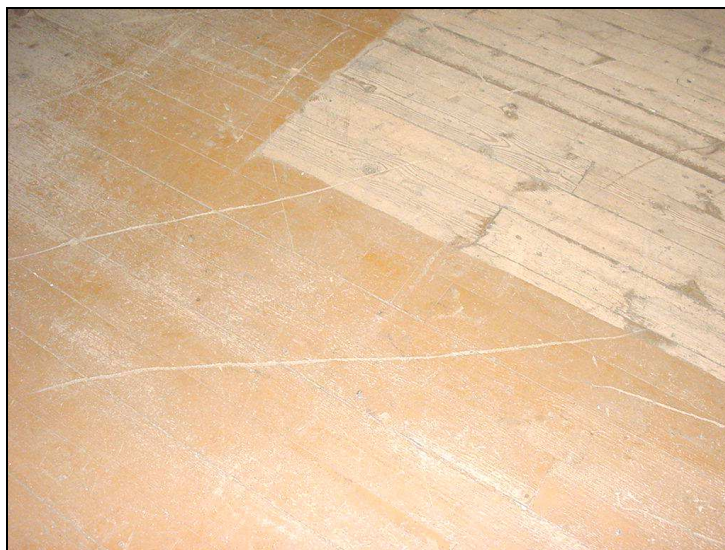
Figure 3: Flaking PCB-containing paint from a wooden floor of a military building (Kuusisto et al. 2006-a)
