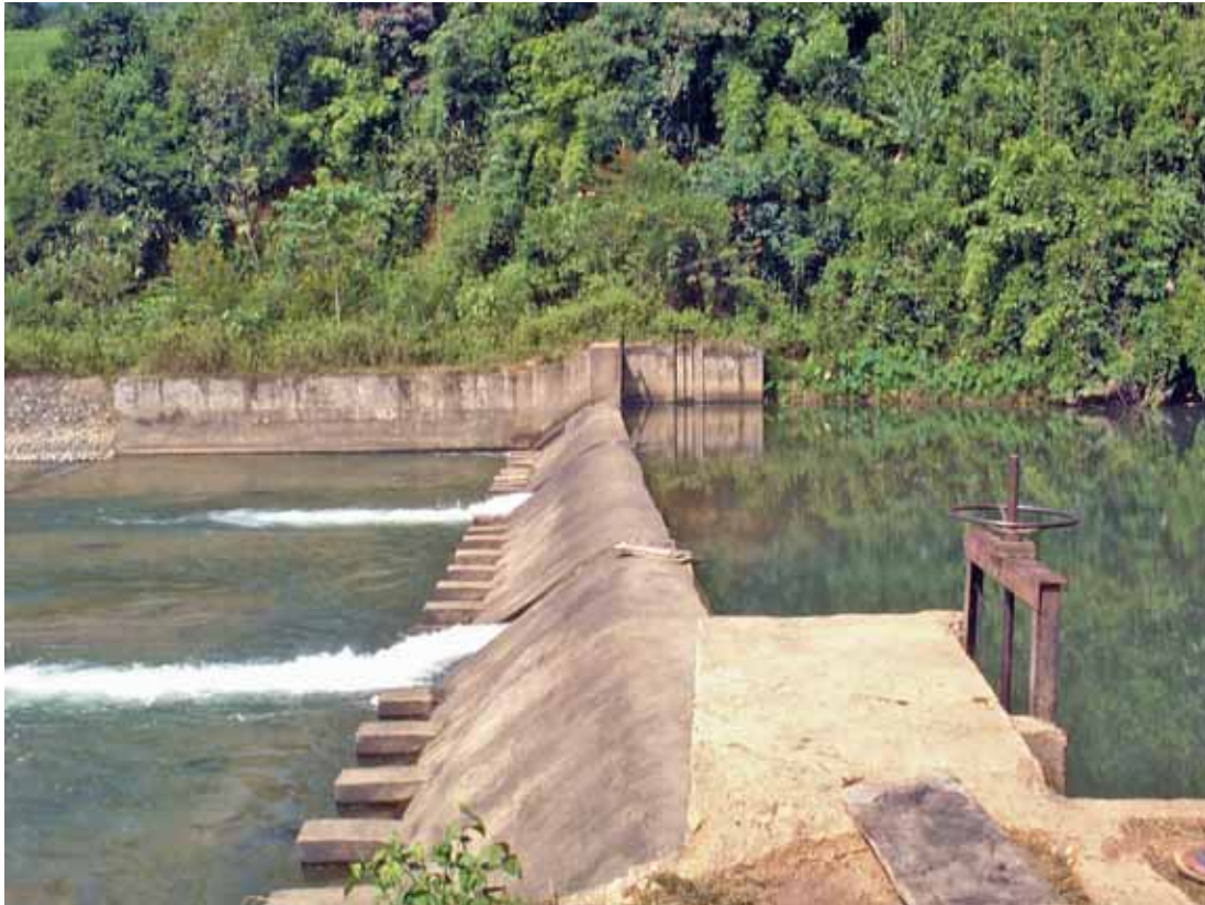
Figure 13: Through the CMI Project, concrete weirs were constructed to replace earlier wooden structures in Vang Vieng (photo taken by Sari Jusi in November, 2004)
