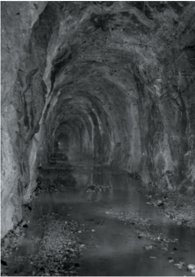
Figure 2. The 120-km long Päijänne Tunnel in 1977. Since 1982 it has supplied raw water to the Greater Helsinki Area, Finland including the Tuusula region. (Photo: TSV)
