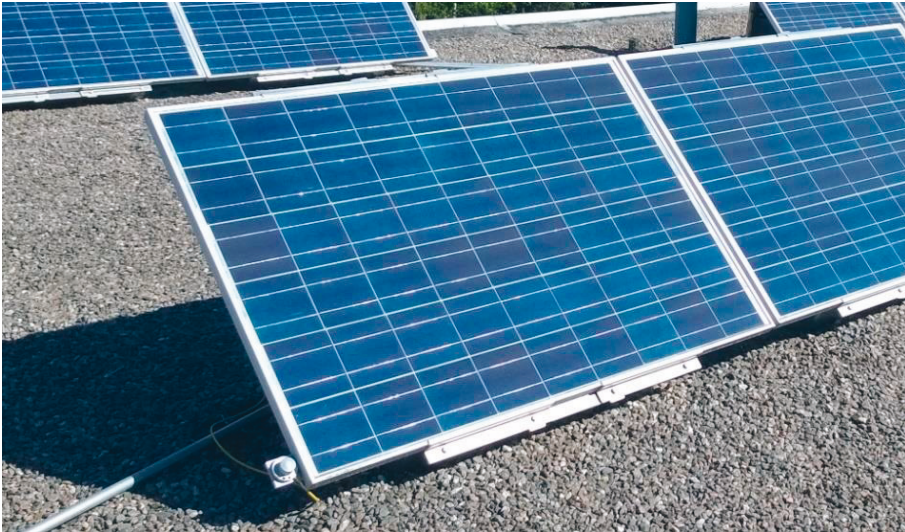
Figure 18. Mounting of the NAPS PV190Kg PV panel and the adjacent S-P Lite 2 irradiance sensor.
