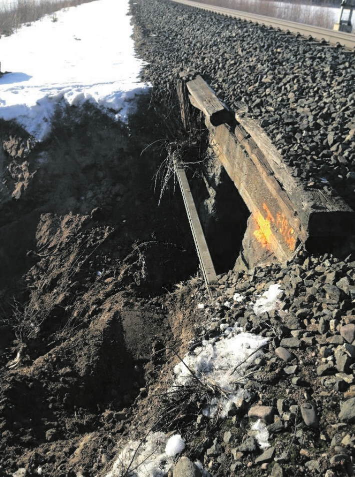
Figure 8. Poor condition culvert with ballast falling over the edge. Photo credit: Mikko Sauni.
