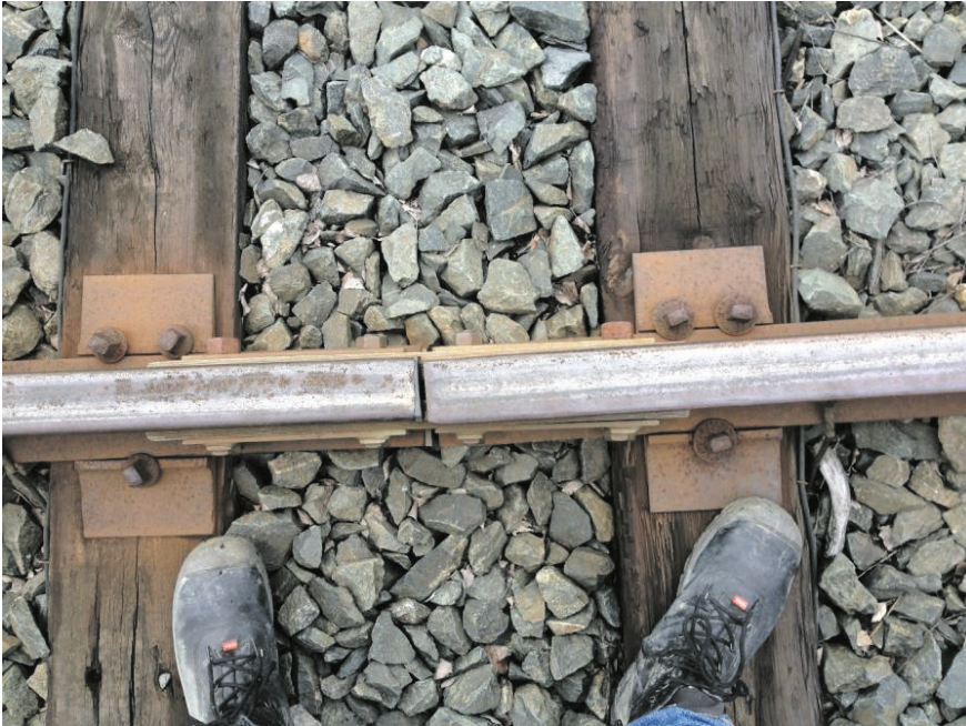
Figure 9. Poor condition insulated rail joint. Photo credit: Mikko Sauni.
