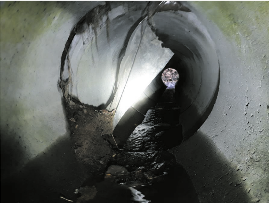
Figure 7. Concrete ring culvert where the rings have been displaced. Photo credit: FTIA asset management registry (Täitorakennerekisteri).
