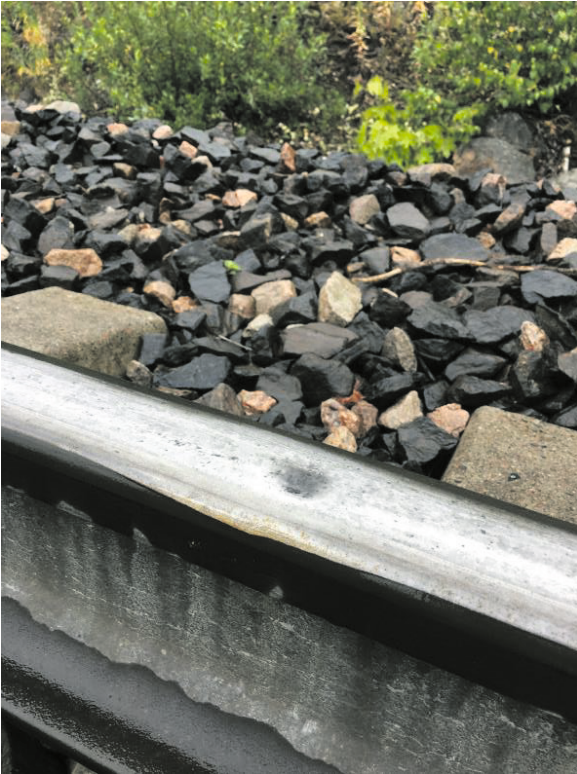
Figure 10. Rail squat defect. Photo credit: Mikko Sauni.
