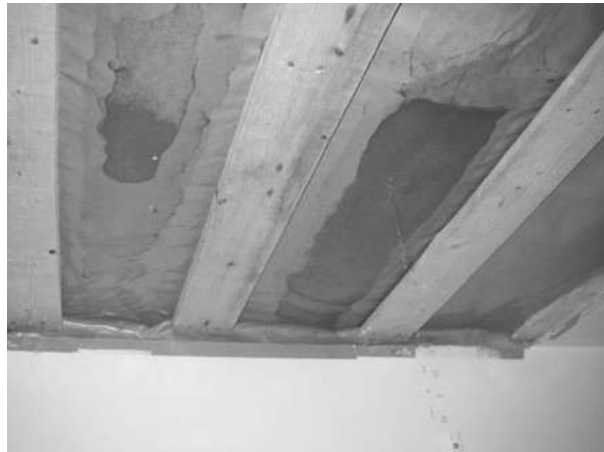
Fig. 4 Example of leak in a roof assembly detected during a moisture performance assessment
