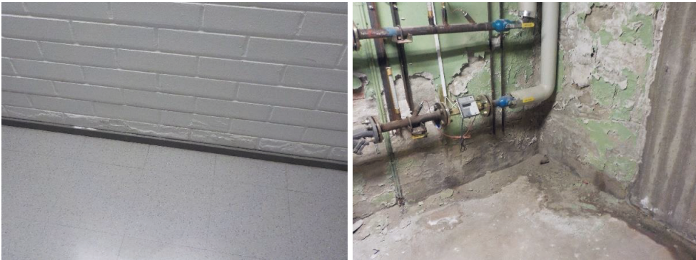
Figure 33. Examples of moisture and mould damage in a masonry wall and in a wall in soil contact.
