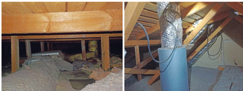
Figure 30. Inside the flat roof (left picture), there is not much space for a condition inspector to check the whole structure, so the reliability of detecting damage is lower than in ridge roofs.
