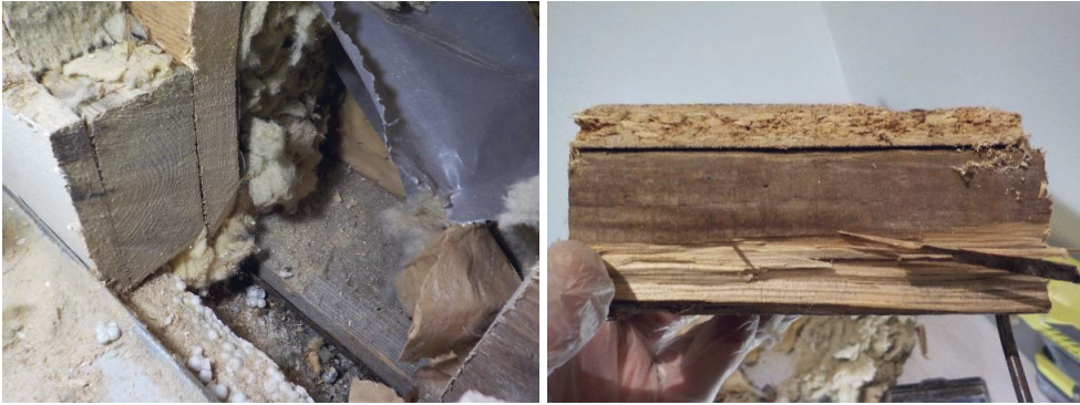
Figure 32. Dismantling of structures is usually necessary to detect moisture and mould in timber-frame buildings.
