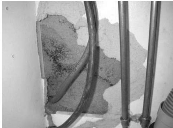
Fig. 3 Example of visually observed mould damage to a chipboard structure
