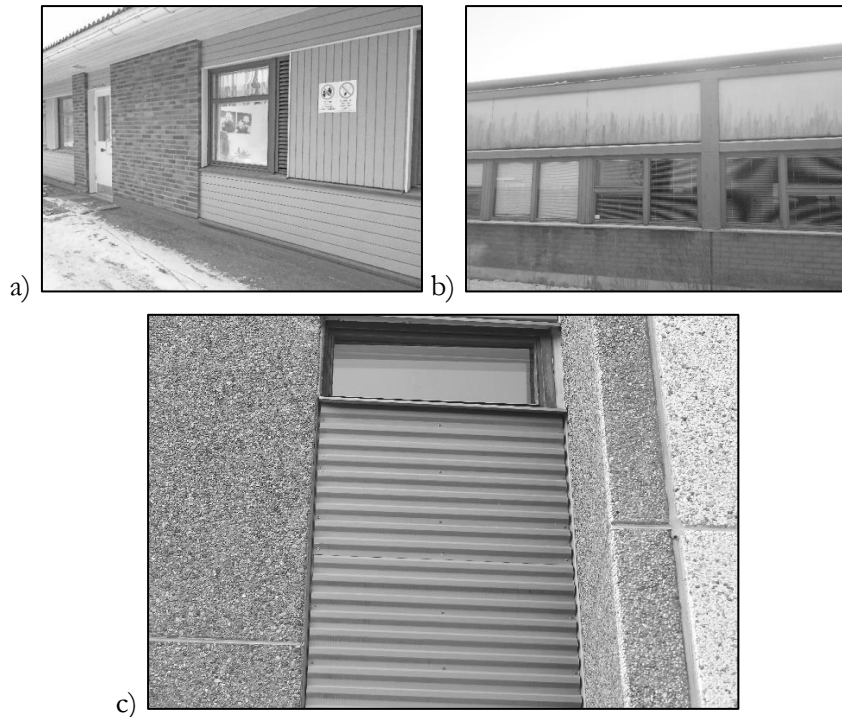
Figure 21. It is very common for façade material to vary in Finnish public buildings, especially around the windows. These examples include changes between a) masonry and wooden panels, b) masonry and a ventilated façade based on cement boards, and c) concrete and a ventilated façade based on metal panels.
