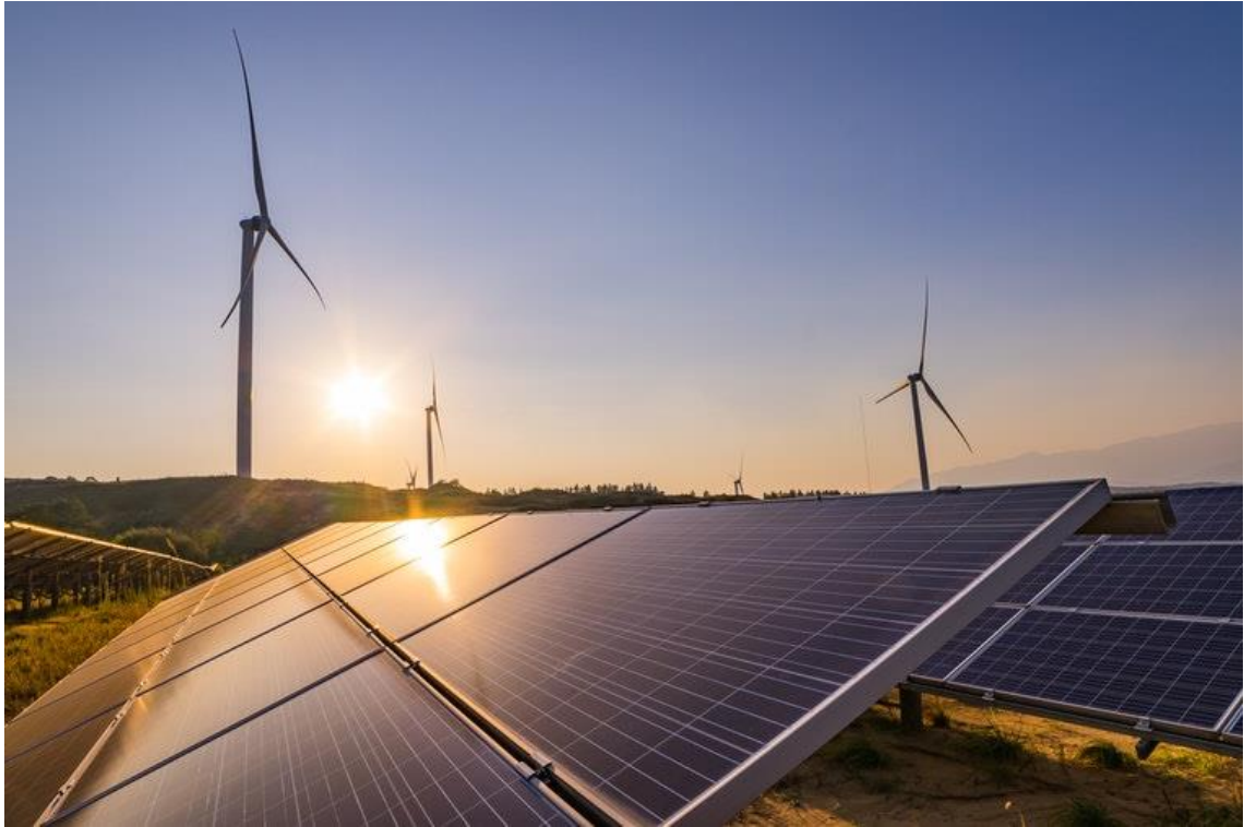
Figure 3: Solar PV panels [3]
