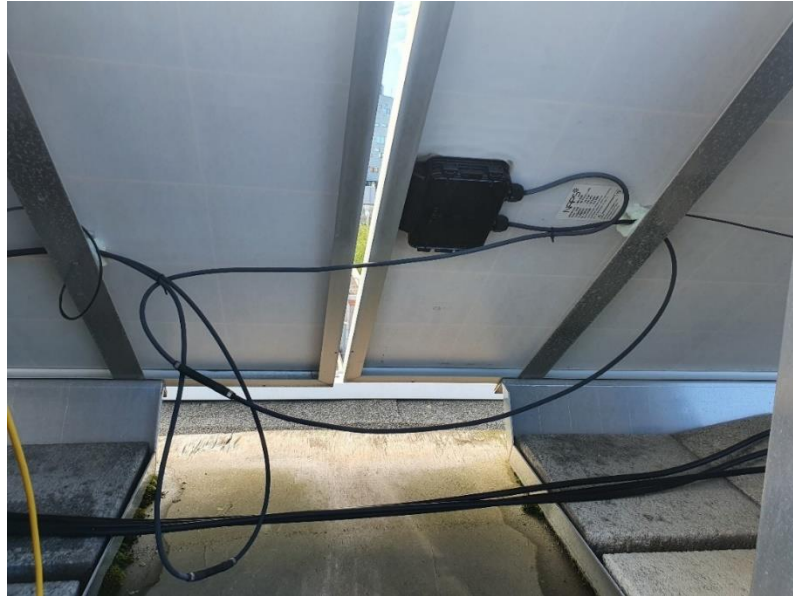
Figure 5.20. Leftmost PV module of the first row in short circuit condition.
