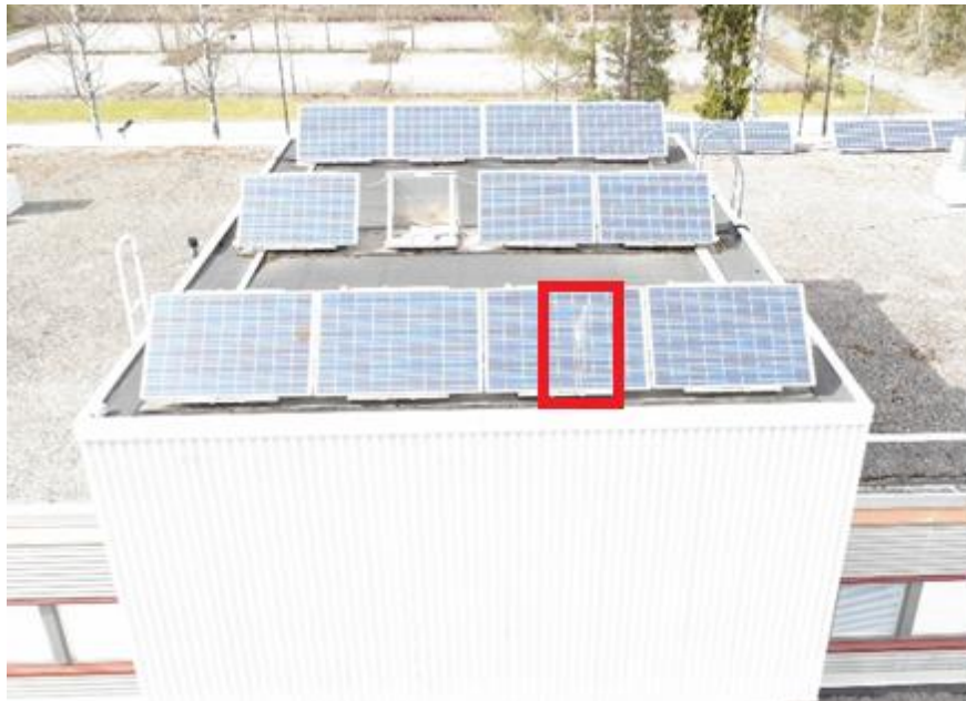
Figure 5.22. Visual image of the uppermost rooftop modules with accumulation of soiling.
