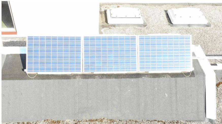
Figure 5.6. Visual image of the leftmost modules of the string 2.
