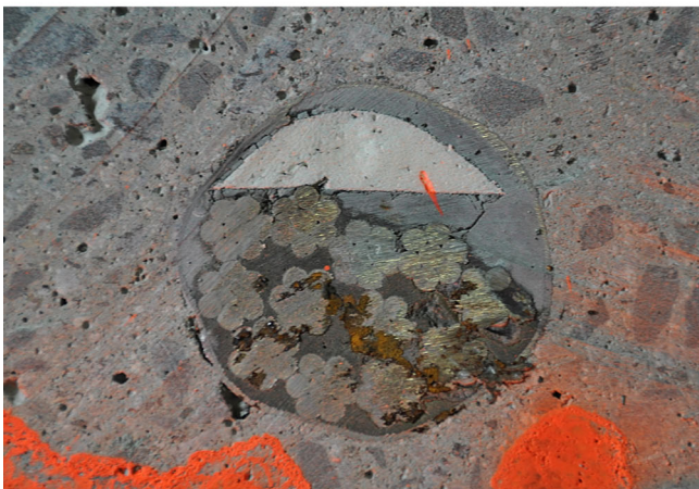
FIGURE 6 Sawed cross sections of test beam 5. In the middle of the beam (left), 300 mm from the end of the beam (right)
