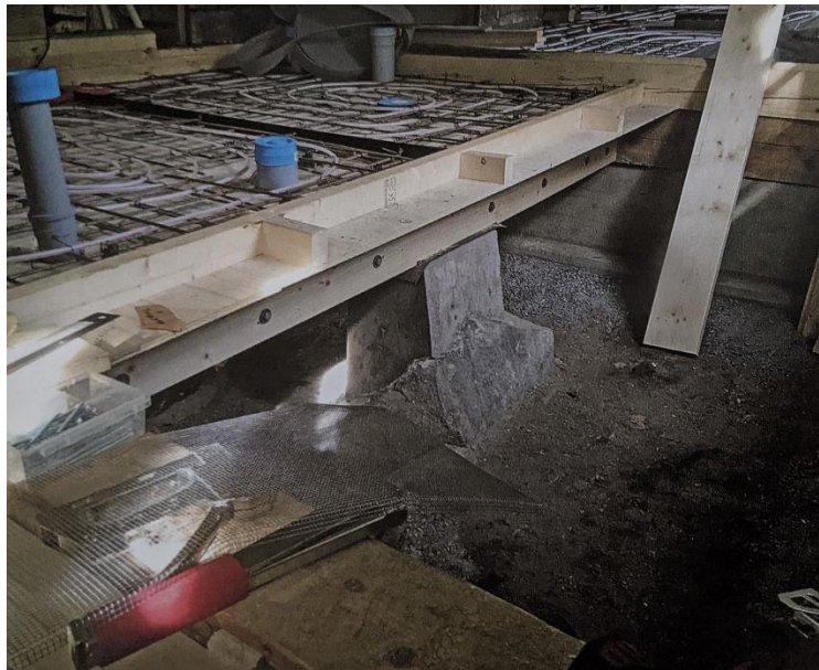
Implementation of new bathroom floor. Construction begins with floor structure, piping and insulation and floor heating pipes if needed. From the publication of Rakennuserienteen Ystävät Ry: Hygienic Facilities in Old Houses
