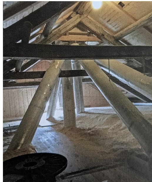
New exhaust pipes taking air from rooms throughout the chimneys. From the publication of Rakennuserienteen Ystävät Ry: Hygienic Facilities in Old Houses
