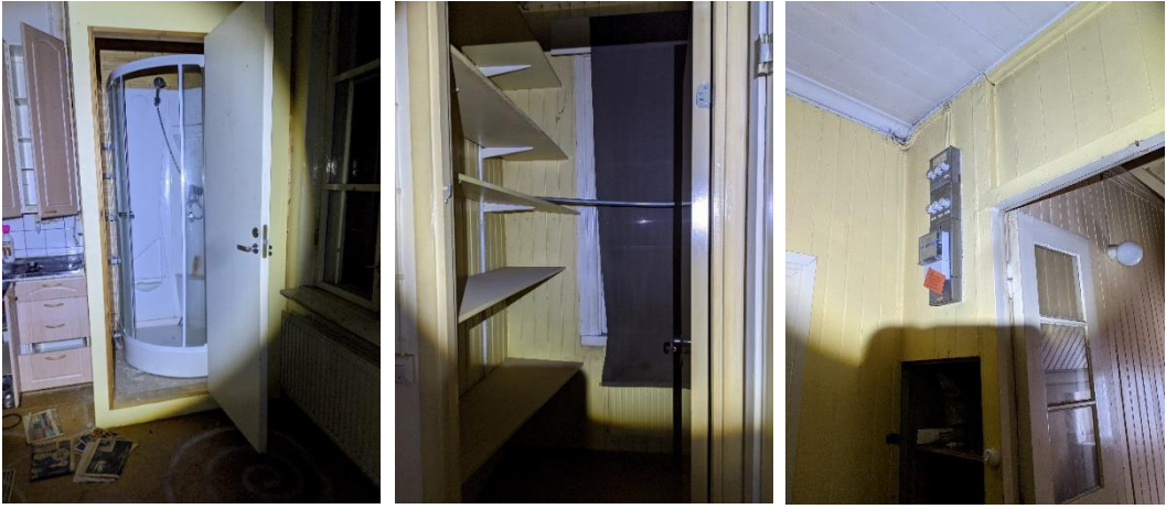
Improper additions from the previous renovations.
