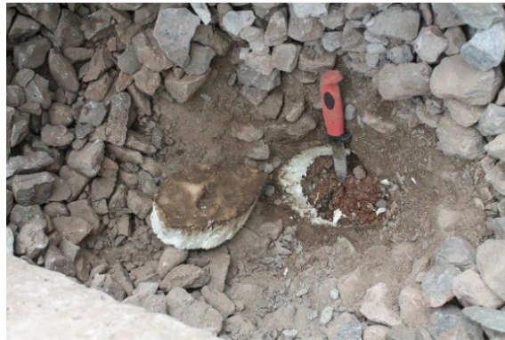
Fig. 5. A frost insulation board underneath ballast at sample point 216+068. Photo credit: Toni Saarikoski.
