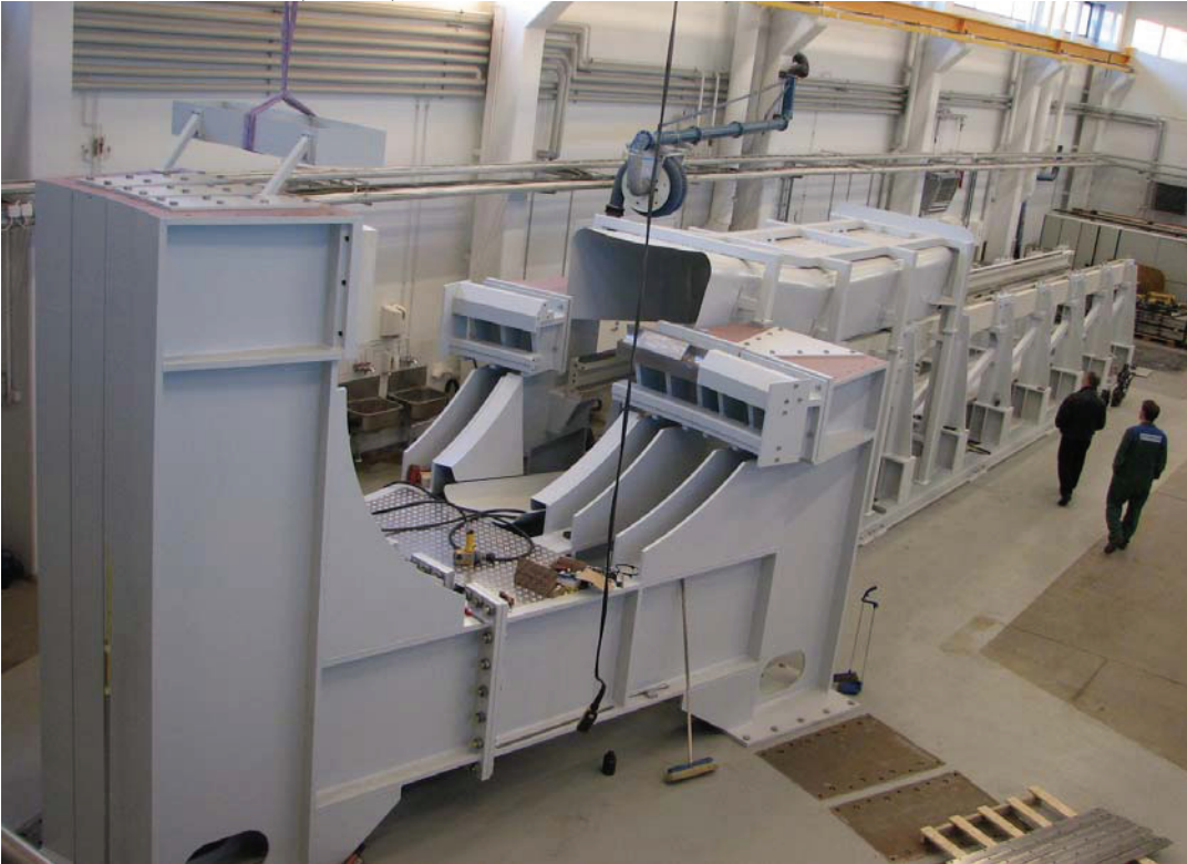
Figure 3. DRM including the maintenance tunnel and reactor section under construction in VTT
