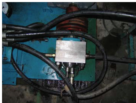
Fig.22 Installation situation of the pump
