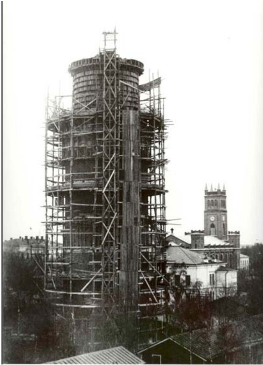
Figure 4. The water tower of the first water works under construction in 1914. It has been in operation since its completion.
