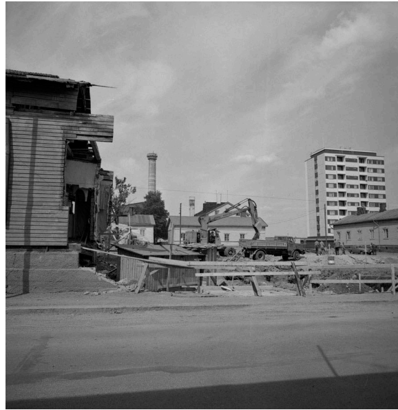
Figure 2. The wooden district of Amuri (Tampere, Finland) under demolition in 1970. Photograph by Ensio Kauppila / Vapriikki Photo Archives.
