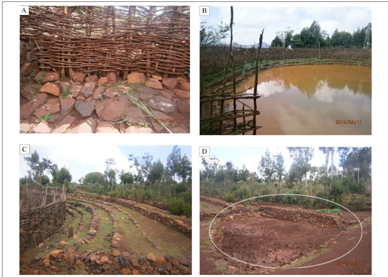
Figure 4. (A) Wooden mesh to filter debris coming to the pond, (B) fenced pond, (C) outside terracing to protect silt from side of the pond, and (D) stilling basin that settles silt coming in with flood before entering the pond.
