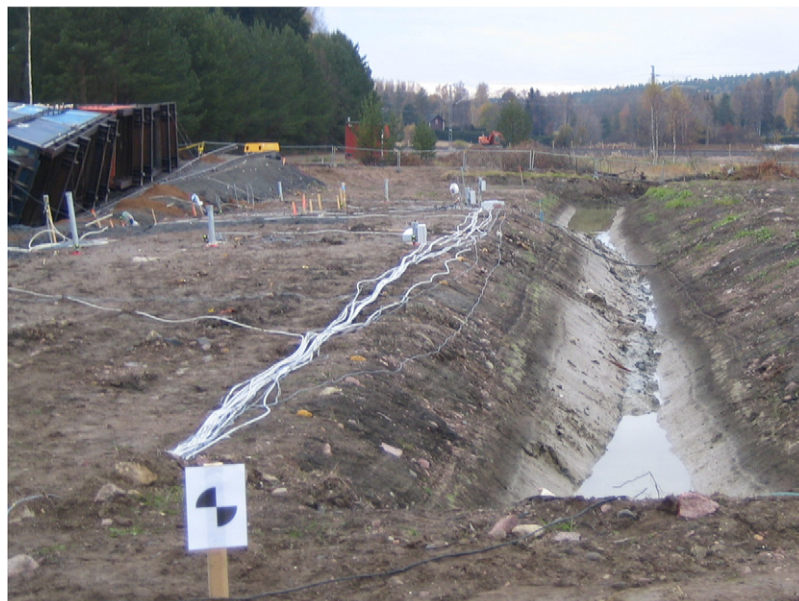
Fig. 10. Post-failure photograph of the embankment failure area at the Perniö test site
