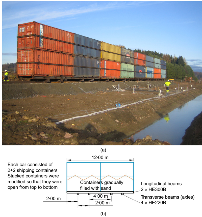
Fig. 7. (a) Test site and containers before loading; (b) container layout used to simulate train car loading pattern
