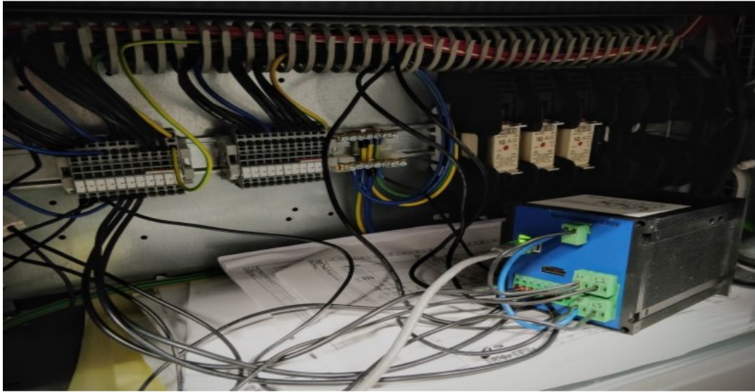
Figure 6. Laatuvahti 3 installed in the main distribution room at pilot building [18].
