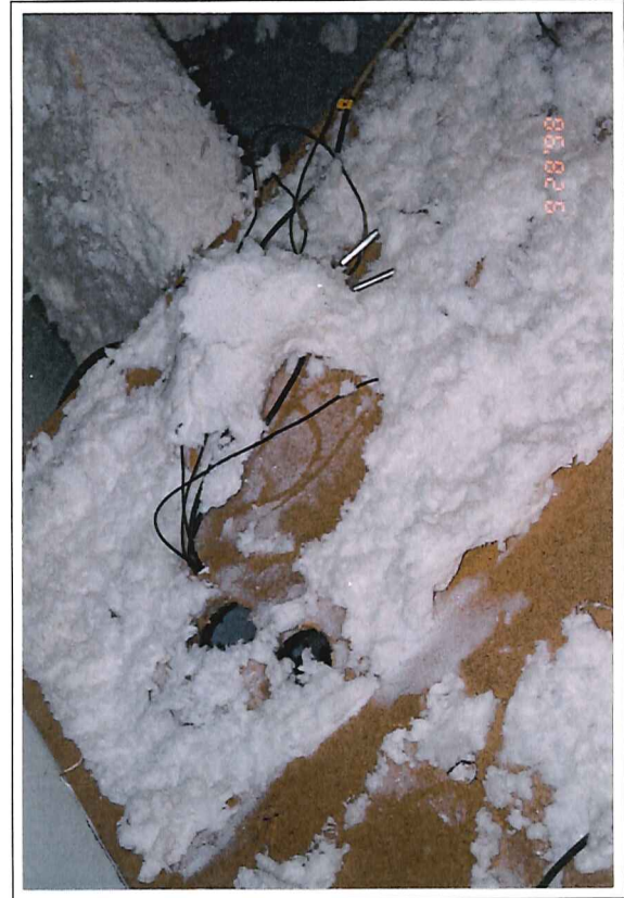
III 8. In Test Wall 8 the thermal insulation frozed to the windshield almost everywhere (rotate to view).
