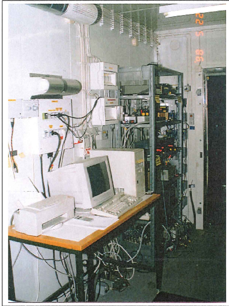
Figure 2.3 Measurement and control instruments of the test equipment.
