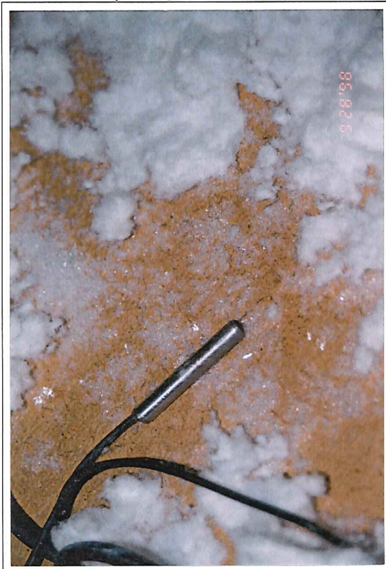
III 7. In Test Wall 8 heavy condensation occurred on the backside of the windshield (rotate to view).
