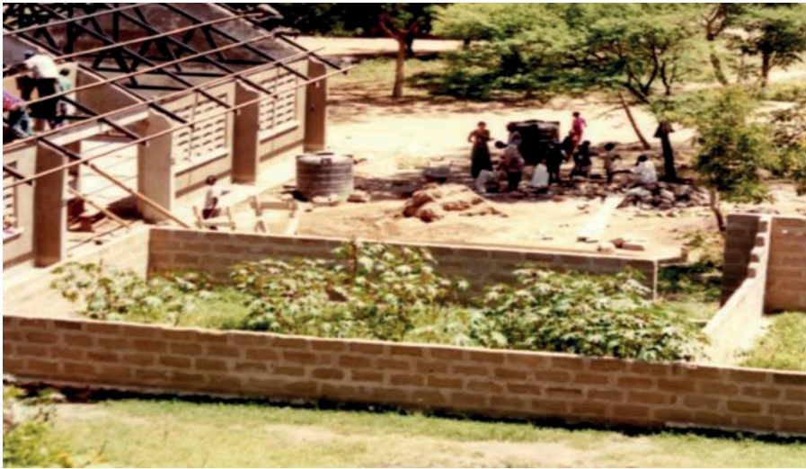
Figure 8. A school construction, the workplace of one MHCC carpentry and joinery graduate interviewed (Pylvänäinen 2001)
