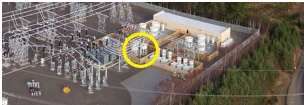
Figure 5. A main reactor SVC in Beaulieu, United Kingdom, main reactor marked with a yellow circle, adapted from [16].
